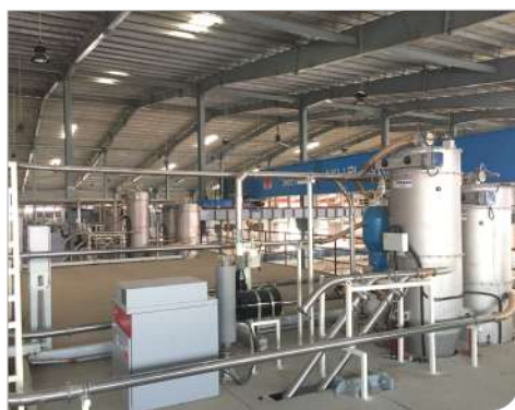
Vacuum Conveying System
