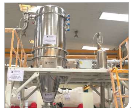
Vacuum Conveying System
